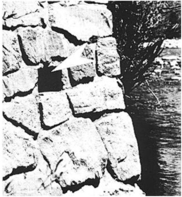
Figure 3. Cavity in a bridge support which contained a Dipper nest.
