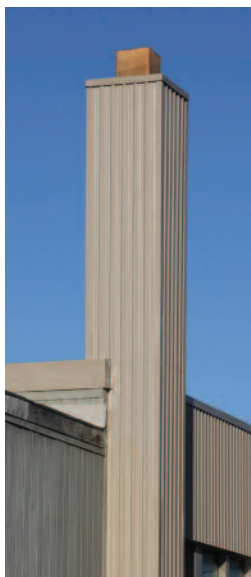
Figure 2. A swift chimney not long after a November 2009 certificate presentation, showing upper portion of the shaft in very poor condition, with missing mortar, loose bricks and lime deposits, London, Ontario, 21 April 2010.
