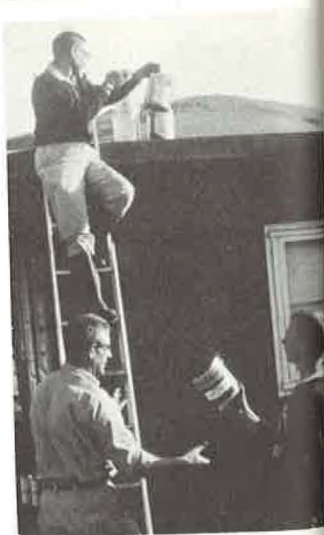
At right - Roofing compound is handed from Ted to Dick and on up to Manuel Morris, Acting Regional Chief of Lands, San Francisco office, a volunteer worker and a bander (Photos by Frank P. Frazier)
