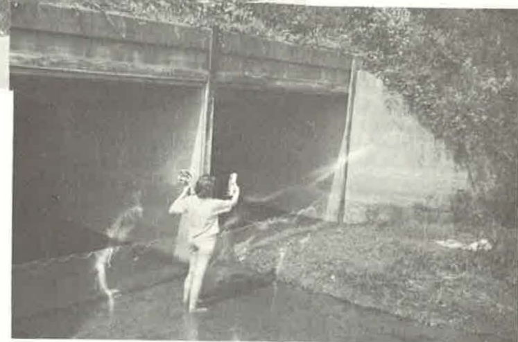
Note framework around entrance and hardware cloth at the bottom of the culvert
