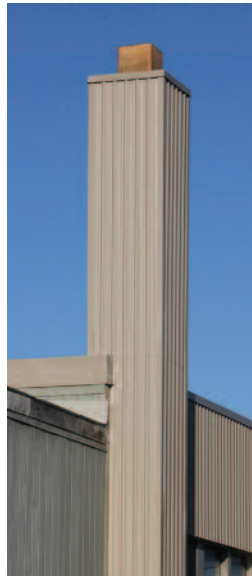
Figure 2. A swift chimney not long after a November 2009 certificate presentation, showing upper portion of the shaft in very poor condition, with missing mortar, loose bricks and lime deposits, London, Ontario, 21 April 2010.
